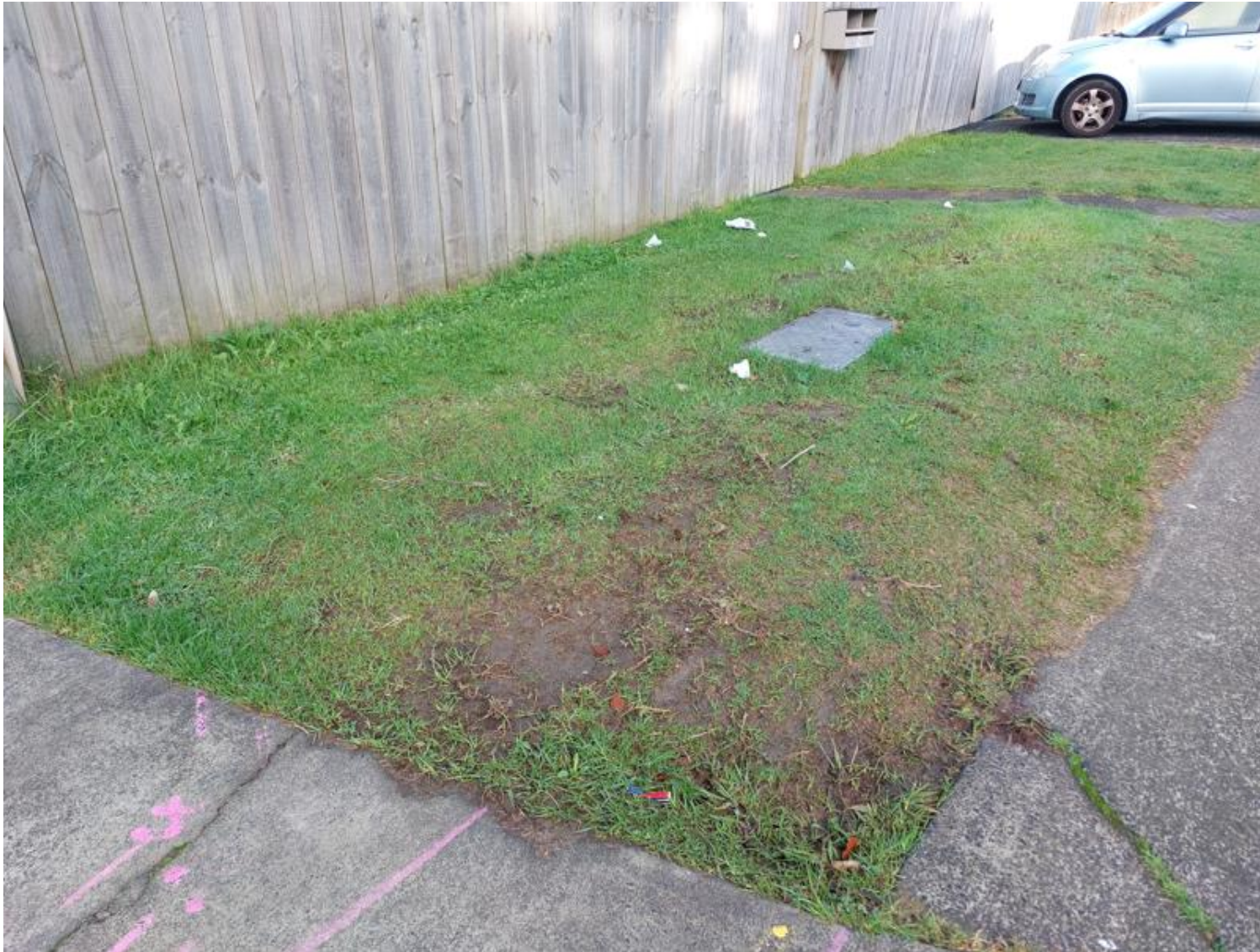
Image 7.4 – Damaged road berms
