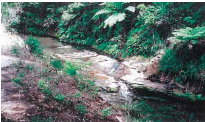
Cuts in the Stream Bank - Swanson's Holding Dam, Swanson Stream, between Woodside Reserve and Helena Park
