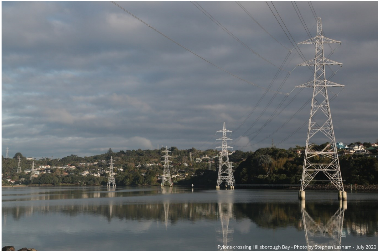
Figure 1 - Pylons crossing Onehunga Bay to Hillsborough
