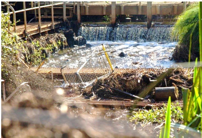
Debris and materials blocking pipe network
