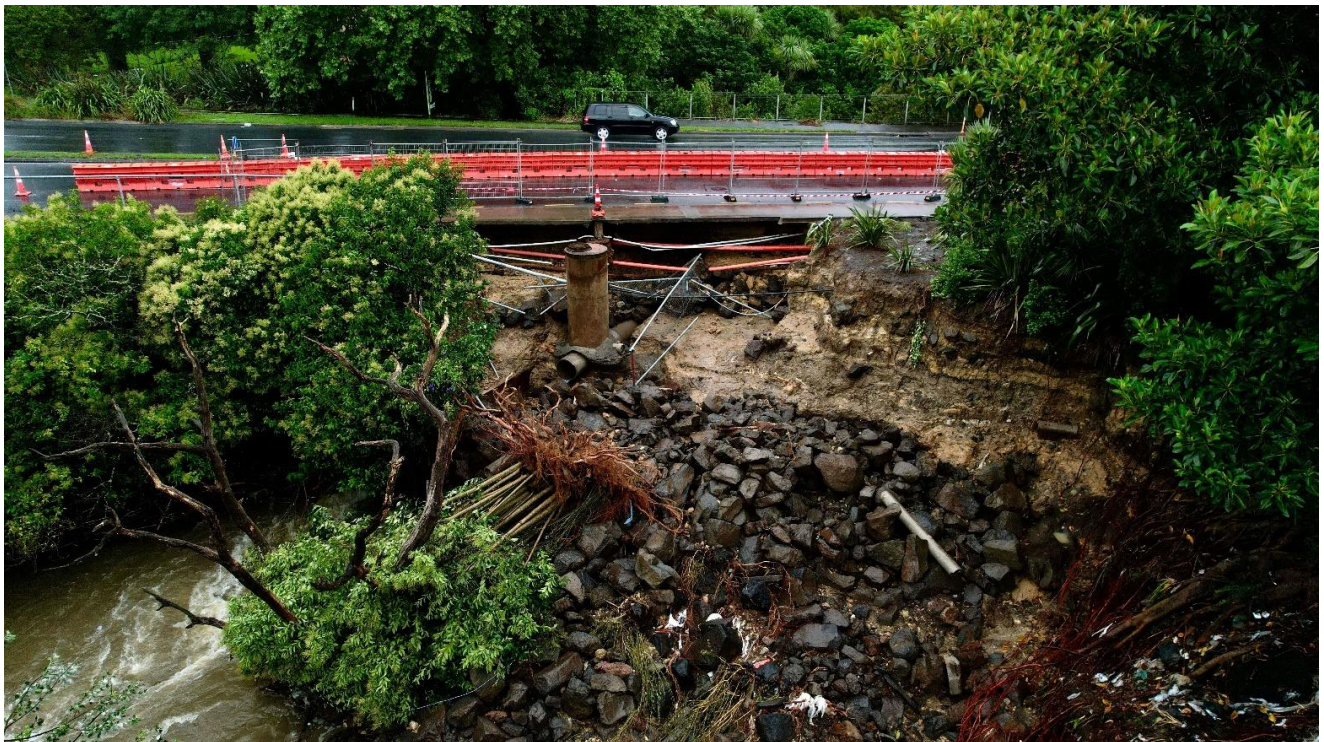
Damage to culvert on Great North Road
