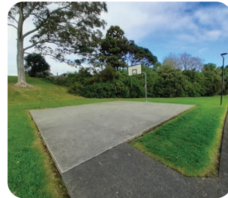
Basketball court with faded markings
