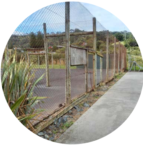
Degraded court edge and fencing
