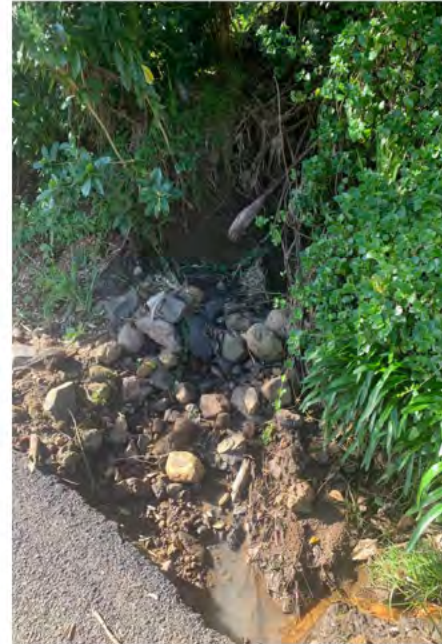
11 Glenesk Rd - significant stream. Culvert across the road does not meet specification
