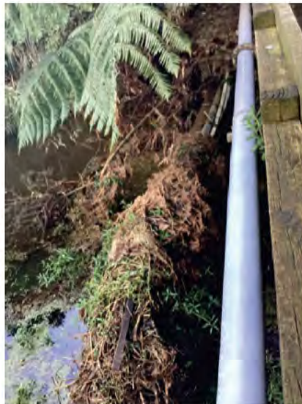
Debris on Pipework & Cables Crossing Coastal Pond
