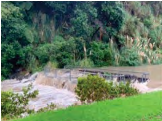
Debris on Tidal Gates blocking Coastal Pond ( this was cleared by local residents)
